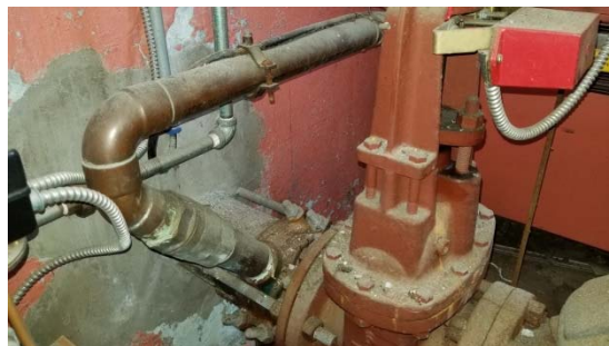
2" Domestic Water Service
