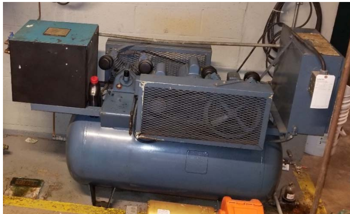
Controls Air Compressor
