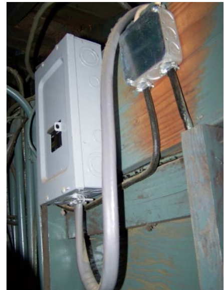
Non-metallic sheathed cable serving circuit breaker, above stage
