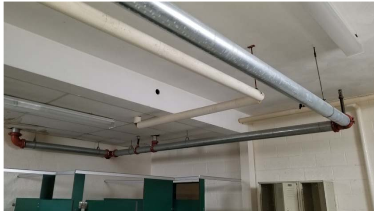
Galvanized Piping with Victaulic Couplings
