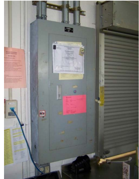
Kitchen panelboard, surface mounted
