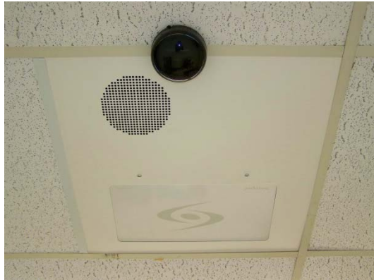
Classroom sounds reinforcement system
