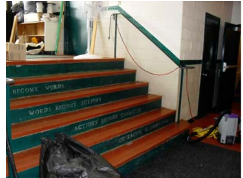
Stair G handrail height and extensions do not meet code.
