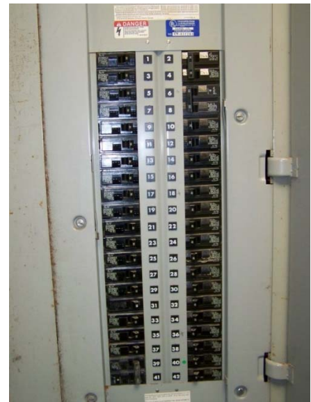
Panelboard L1 located in first floor janitors closet, single phase panelboard
