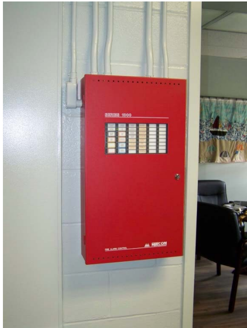
Fire alarm control panel located in gymnasium lobby
