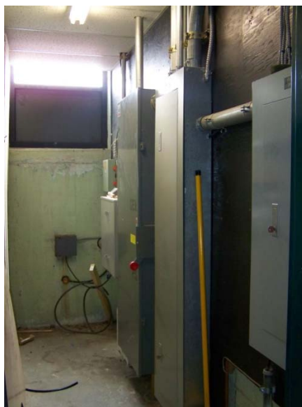
1 st floor, main electrical room
