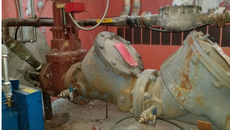
Domestic Water Tap, Shut-off Valve and Backflow Preventer
