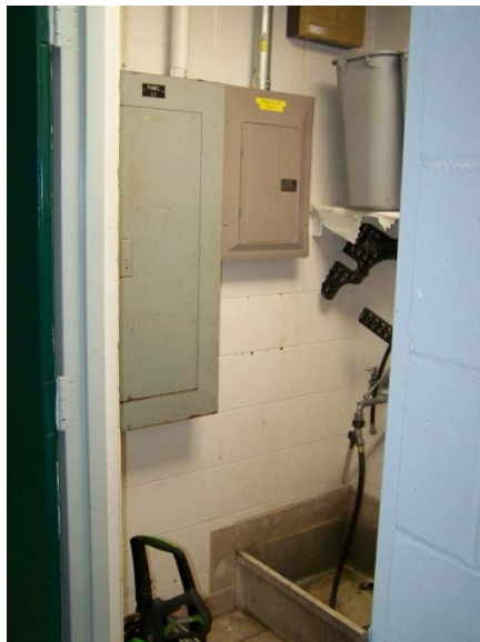
Panelboards in typical janitors closet, code required working clearances do not exist
