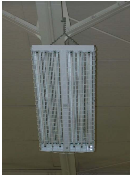
Gymnasium lighting fixture
