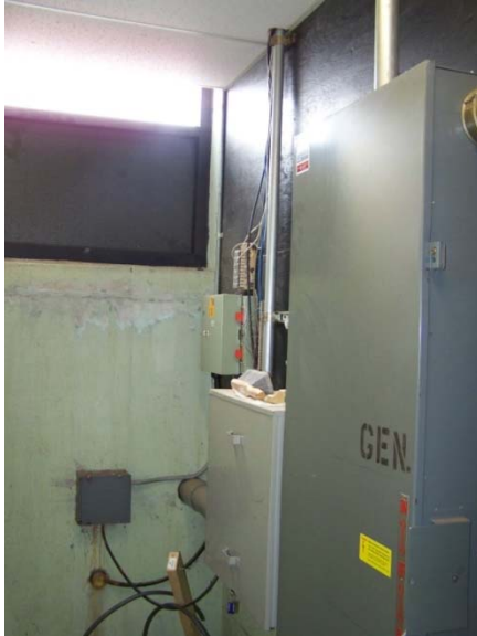
Demarcation in main electrical room
