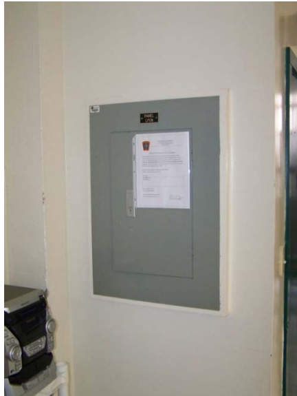
Cafeteria panelboard, semi-recessed
