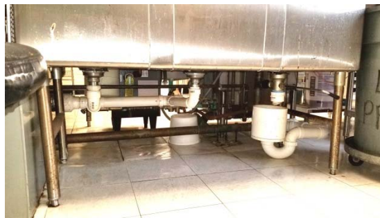
Three Bay Sink Drains
