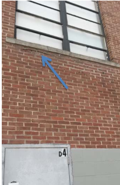
Exterior brick wall with loose mortar joints
