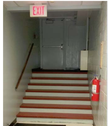
Stair D, needs handrail on right of stair. Note conflict with unit heater.
