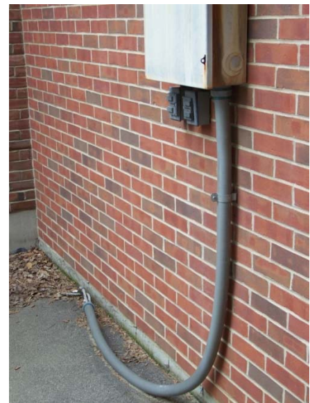
Generator connection box/disconnect with generator umbilical still attached
