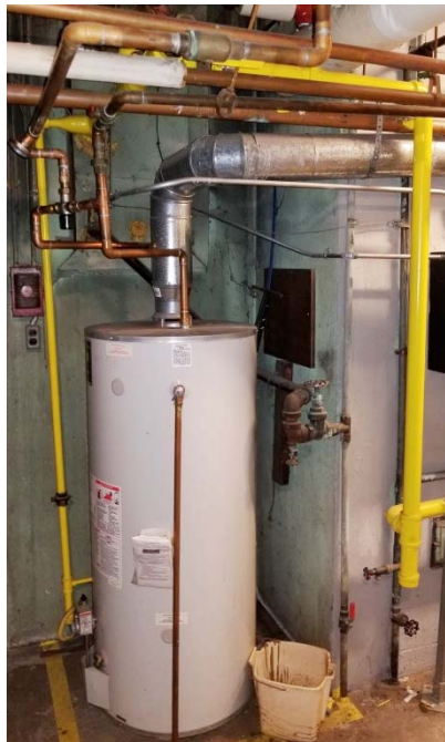
Existing Natural Gas Fired Water Heater
