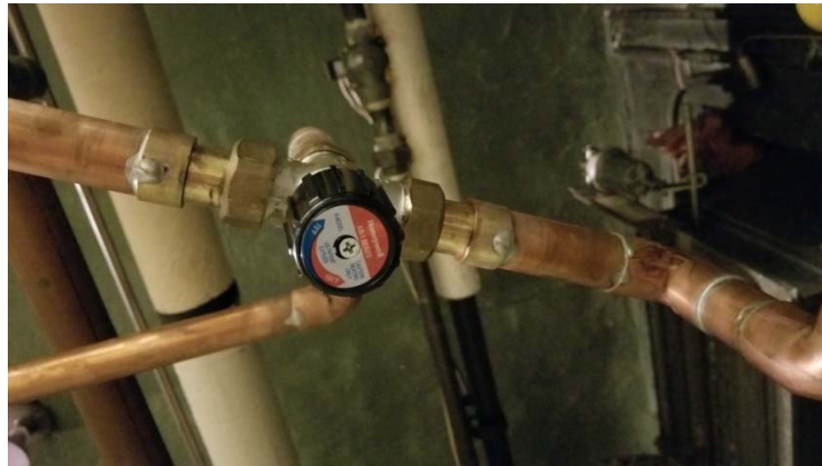
Existing Honeywell Thermostatic Mixing Valve
