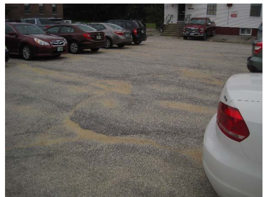
Differential settlement and sediment observed in lot
