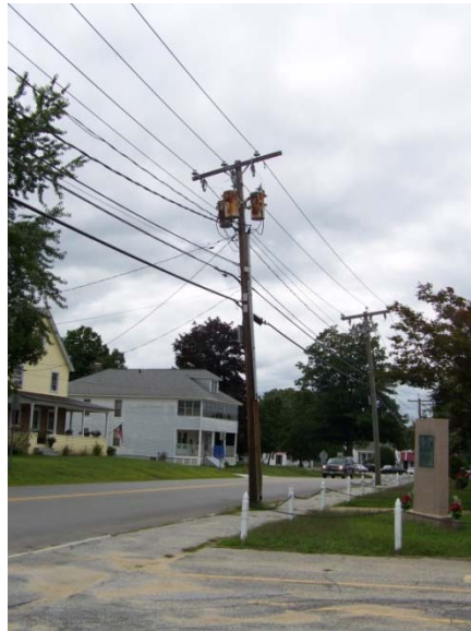
Pole mounted transformers serving St. John the Baptist Church and Armand R. Dupont Middle School
