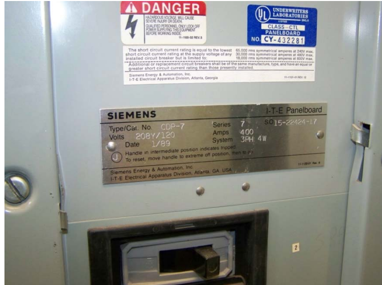
1 st floor, main electrical room, main panelboard MP, manufacturers badge
