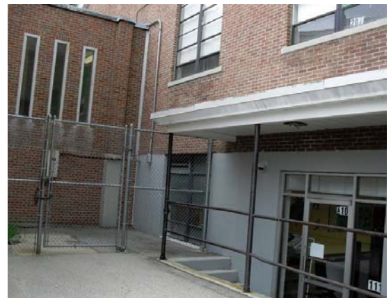
Exterior stairs K need handrails both sides of stair and balusters and guardrail do not meet code.
