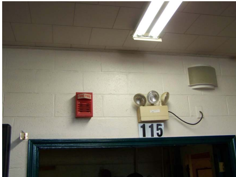
Typical emergency egress / life-safety lighting battery unit
