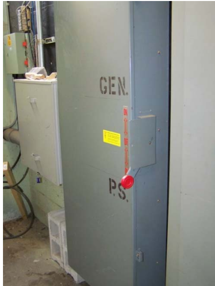
Manual transfer switch (service disconnect) with CT cabinet and feeder from utility on the left, panelboard with overcurrent protection at right of transfer switch
