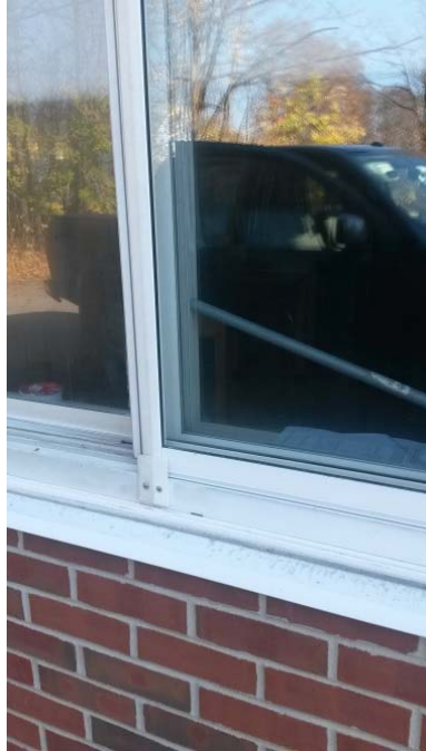
1988 Addition west elevation. Note wood dowel used to secure window due to latch not functioning.
