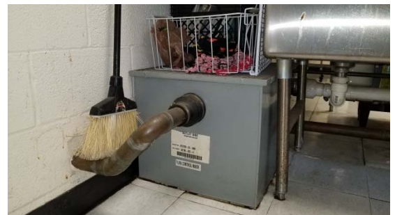
Grease Interceptor Discharge
