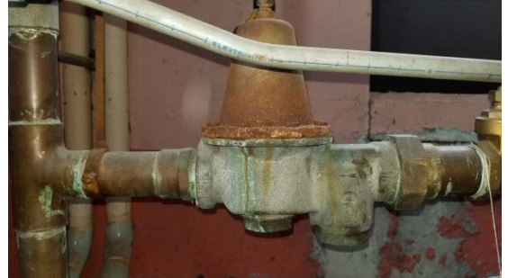
2" Pressure Reducing Valve
