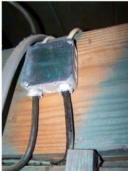
Cloth insulated wiring (black) with non-metallic sheathed cable (white), above stage
