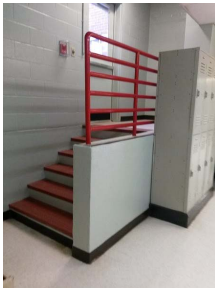
Stair C, needs handrails both sides of stair.
