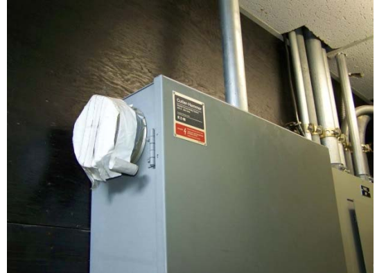
Knockout on transfer switch covered with tape
