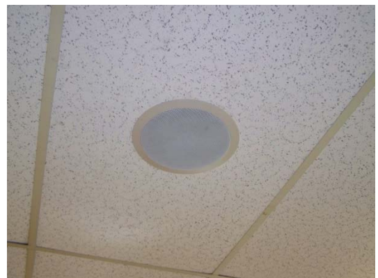
Typical recessed speaker, non-classroom locations
