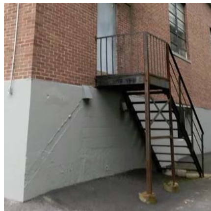
Exterior stair M need handrails both sides of stair and balusters and guardrail do not meet code.
