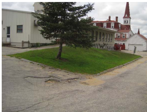
Potholes and sediment observed along access way
