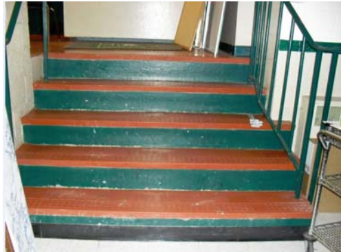
Stair F from Cafeteria #111 iron handrail, balusters and guardrail do not meet code.(Stair E similar)
