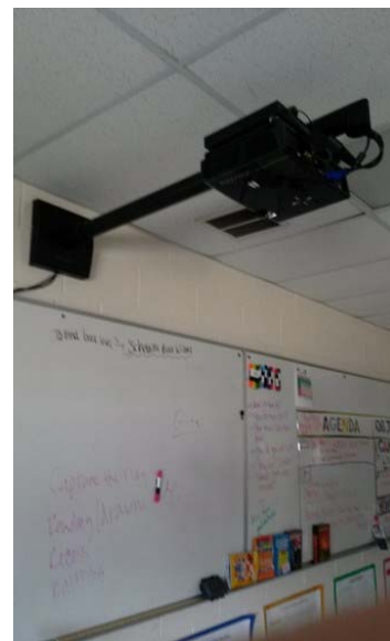
Wall mounted projector with marker board
