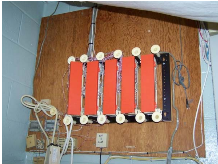
Backboard in administration with phone system punch down blocks
