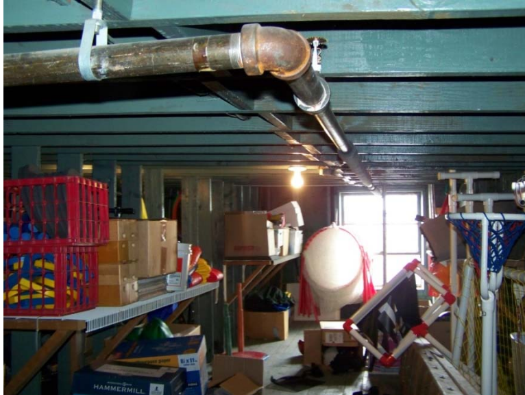
Incandescent lighting in attic space above stage
