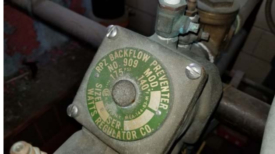
2" RPZ Backflow Preventer
