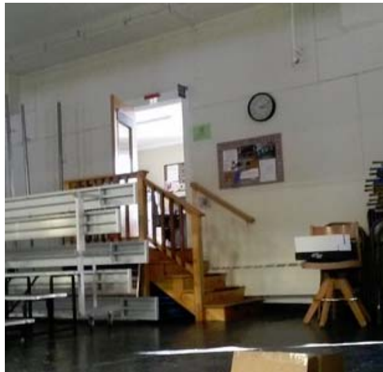
Stair L, wood stair handrail, balusters and guardrail do not meet code.
