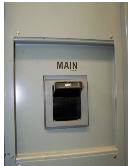
Main panelboard MP main circuit breaker, first overcurrent protective device downstream of the manual transfer switch
