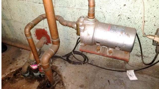
Sump Pump for Kitchen
