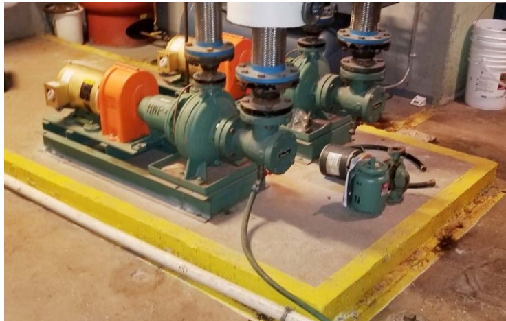
Hot Water Pump
