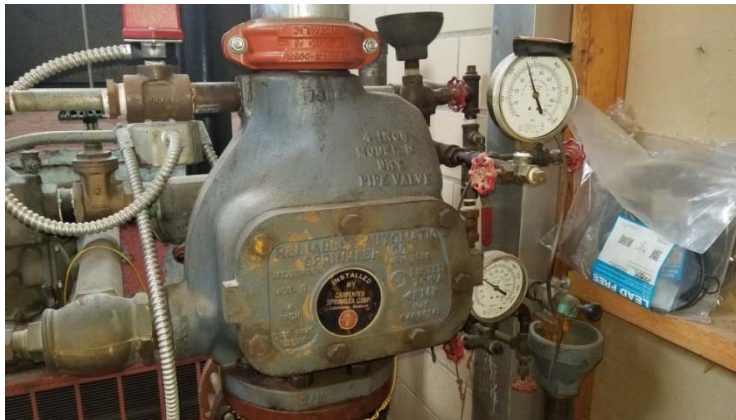
Dry Alarm Valve
