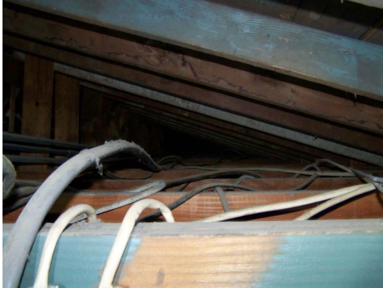
Mixture of non-metallic sheathed and cloth insulated wiring above stage
