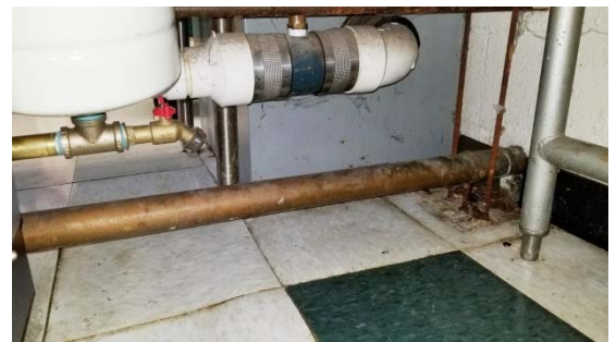
Copper Dishwasher Drain
