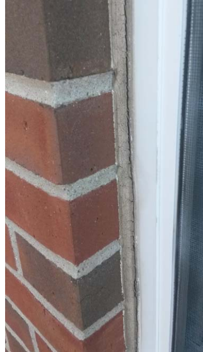
Same window, noting caulking failure.
