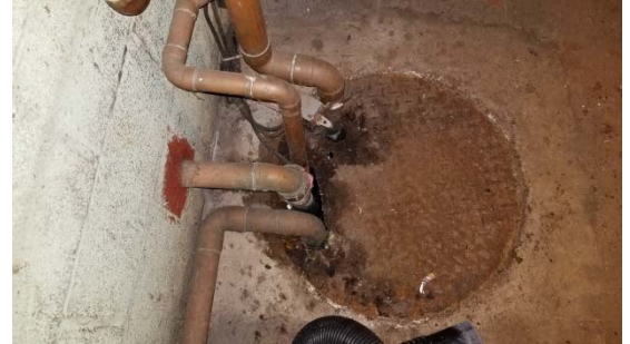
Sump Pump for Kitchen
