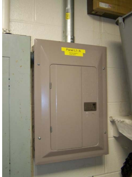
Panelboards have been added next to some panelboards for additional circuit breaker space, this panelboard is adjacent to panelboard L1 in first floor janitors closet
