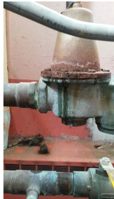
Close-up of Water Leak
