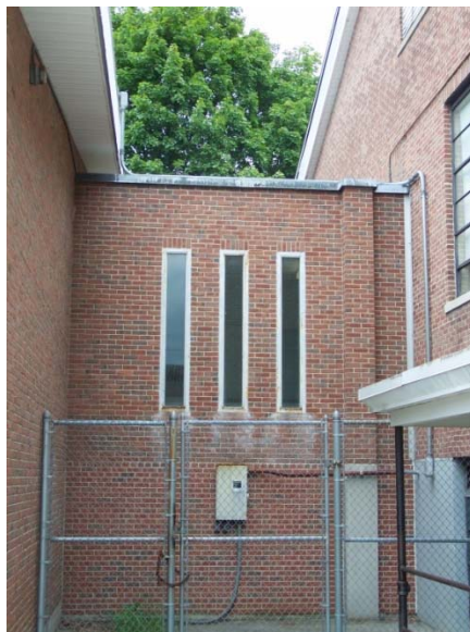
Generator connection box/disconnect
