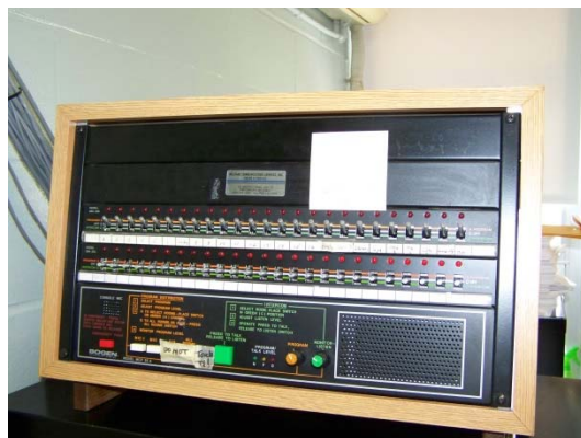
Public address system head end equipment
