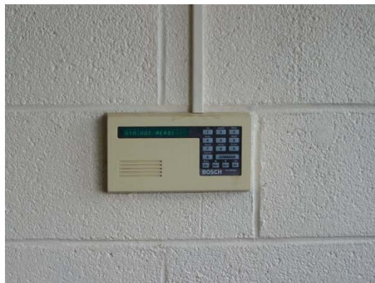
intrusion detection system key pad at main entrance
