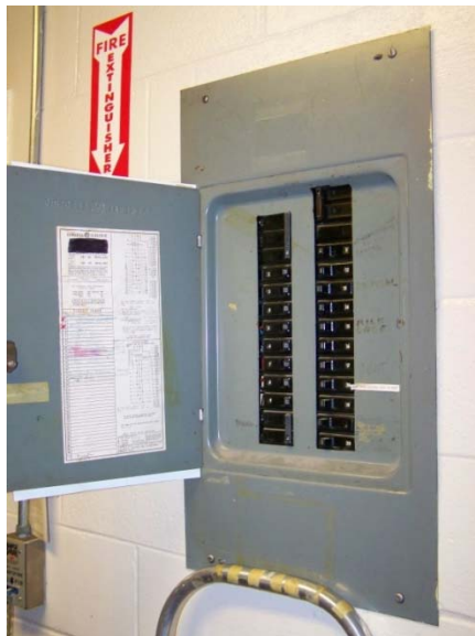
kitchen panelboard #1, recessed, no space remaining and panel cover does not sit tight to wall
