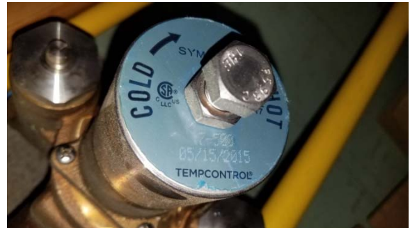
Existing Symmons Thermostatic Mixing Valve
