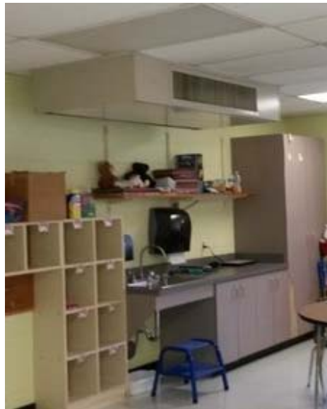
Typical Kindergarten Unit Ventilator
