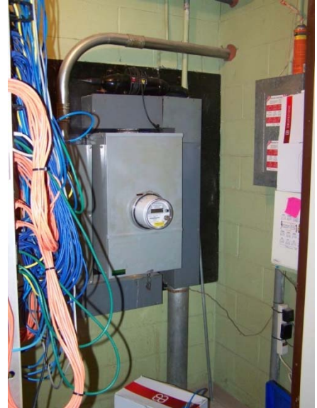
1 st floor, main electrical room, looking right
