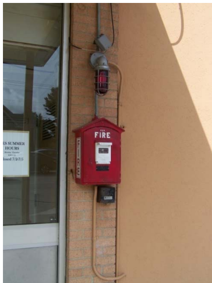
fire alarm system master box, reporting device to the city loop
