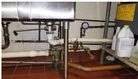
3 Bay Sink and Dishwasher Drainage Piping
