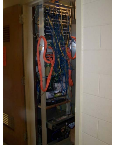
communications rack in main electrical room, inadequate working clearances
