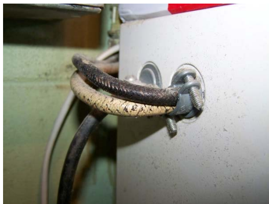
cloth insulated wiring
