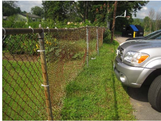
Damaged/rusted fence at southern perimeter
