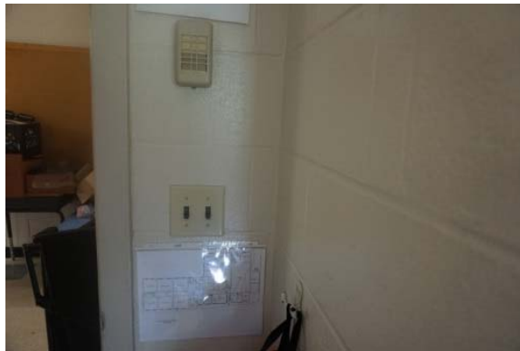
typical classroom switch arrangement
