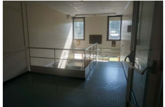
Stair A – handrail termination and guardrail/handrail with balusters along open stair does not meet code.
