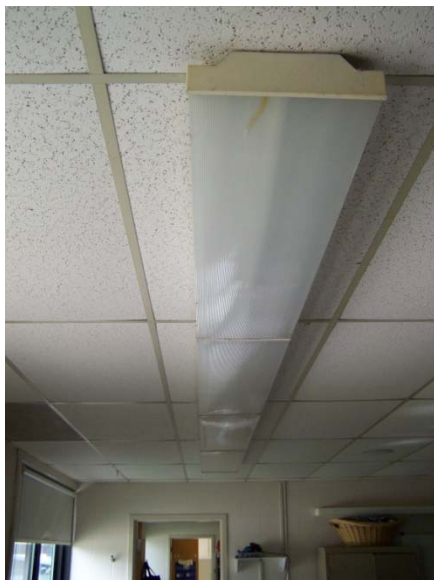
another example of typical classroom lighting
