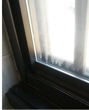
Thermal pane glazing that lost seal
