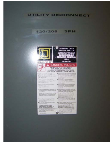
service disconnect, close view
