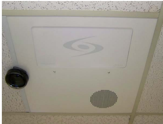
classroom sounds reinforcement system
