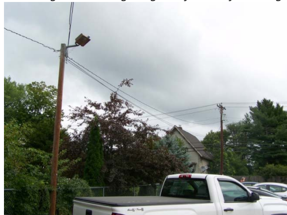
pole mounted flood lighting, utility company leased lights, right side of building
