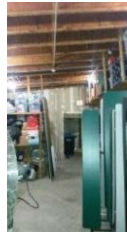
D - View from Storage 140 towards door to Stair D Note wood frame construction.
