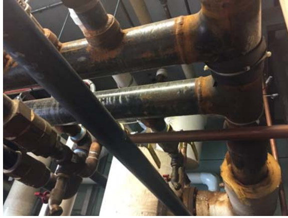
Closed space tee and example of uninsulated pipe
