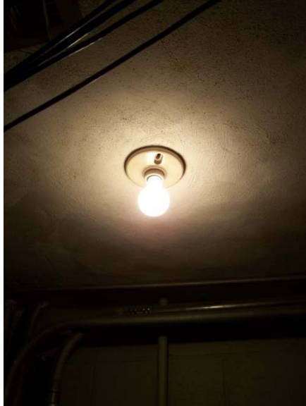
incandescent lighting fixture, main electrical room
