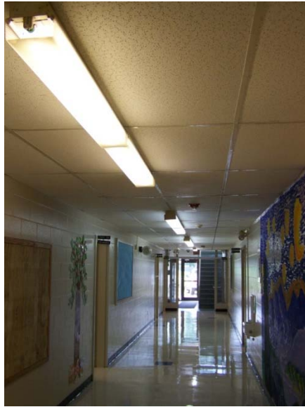
exit sign partially block by surface mounted lighting fixtures
