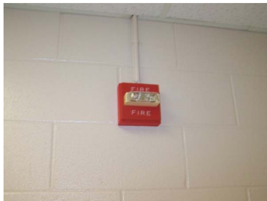
style of fire alarm appliances in the building vary, wall mounted
