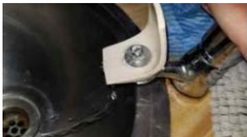
Bubbler not functioning
