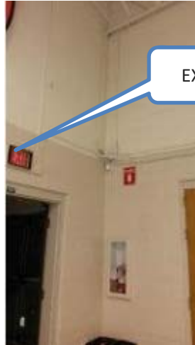
A - Double door viewed from Multipurpose room Note EXIT sign above doors.
