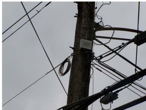
building fire alarm connection to the city loop
