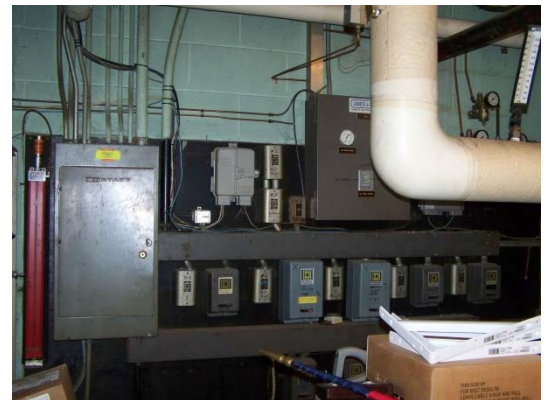
boiler room panelboard with storage impeding access
