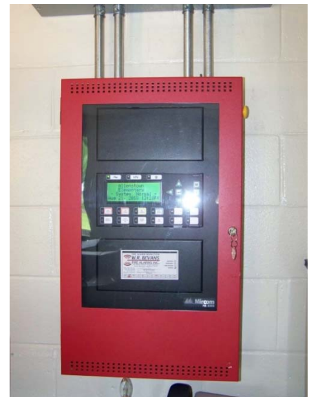
fire alarm control panel located in the main office
