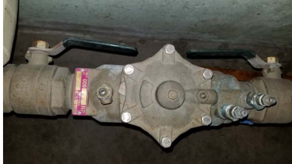
Existing WATTS 009 Reduced Pressure Zone Backflow Preventer
