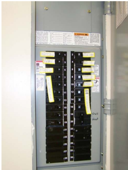
240V/1ph panelboard located in an office in the vicinity of the kindergarten classrooms
