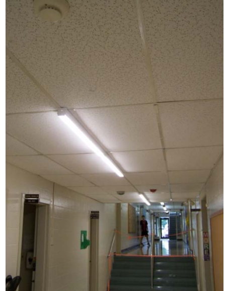
upgraded LED corridor lighting, near main office
