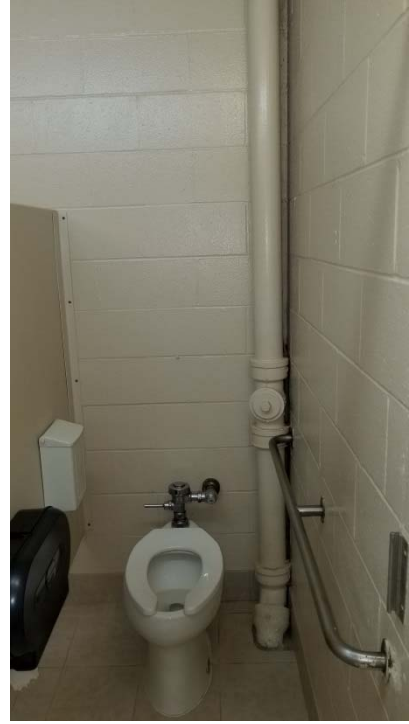
Examples of Cast Iron Piping
