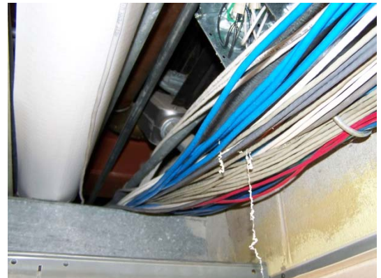
cables above first floor corridor ceiling
