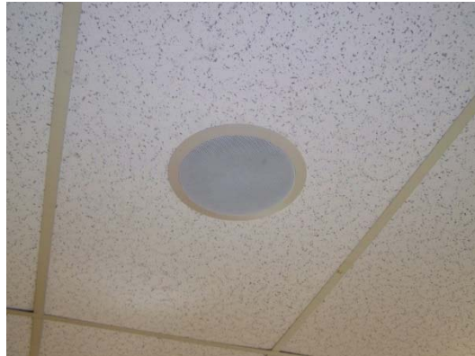
typical recessed speaker, non-classroom locations
