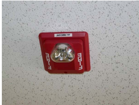
typical ceiling mounted fire alarm strobe
