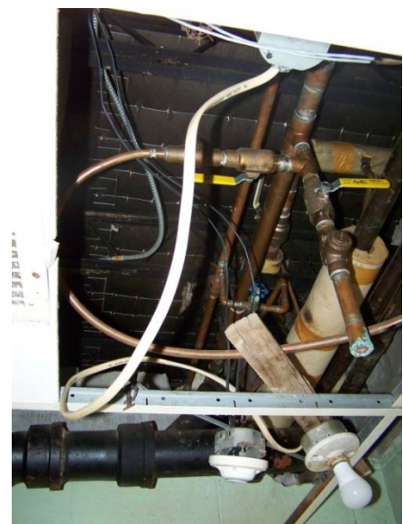
non-metallic sheathed cable – Romex, first floor janitors closet
