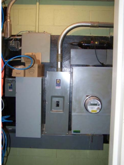
1 st floor, main electrical room, looking straight back
