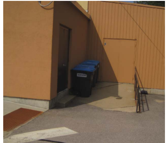
F - Double doors exterior view to Vestibule 139 No landing in front of doors or handrails both sides. If ramp were to be extended to meet code, requirement for landing would interfere with double doors from Storage 138.
