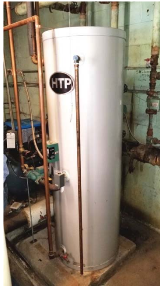
Existing Indirect Fired Water Storage Tank
