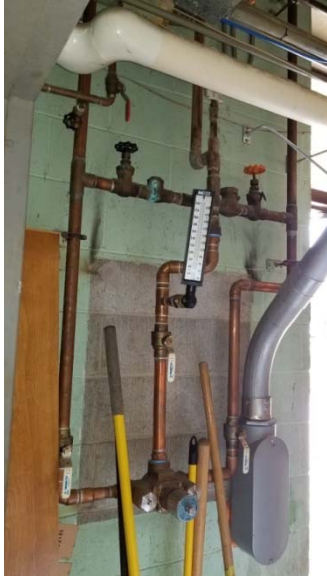
Existing Thermostatic Mixing Valve
