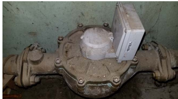
Existing 2" Water Meter
