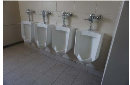
Typical Boys urinals – no ADA code compliant urinals. Require 1 ADA compliant per toilet room in Boys 115 & 213.
