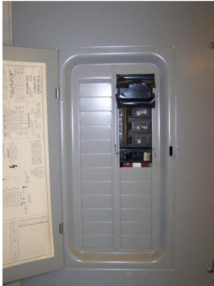
kitchen panelboard, newer panelboard, space remaining for additional circuit breakers, improper filler pieces, exposed parts and appears that a circuit breaker that is not intended for this panelboard installed
