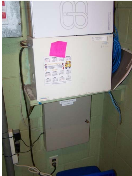
emergency egress / life-safety battery unit plugged in a receptacle, main electrical room
