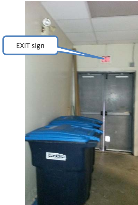
E - Double doors to exterior Note EXIT sign above door.
