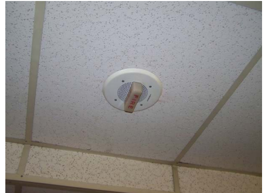
style of fire alarm appliances in the building vary
