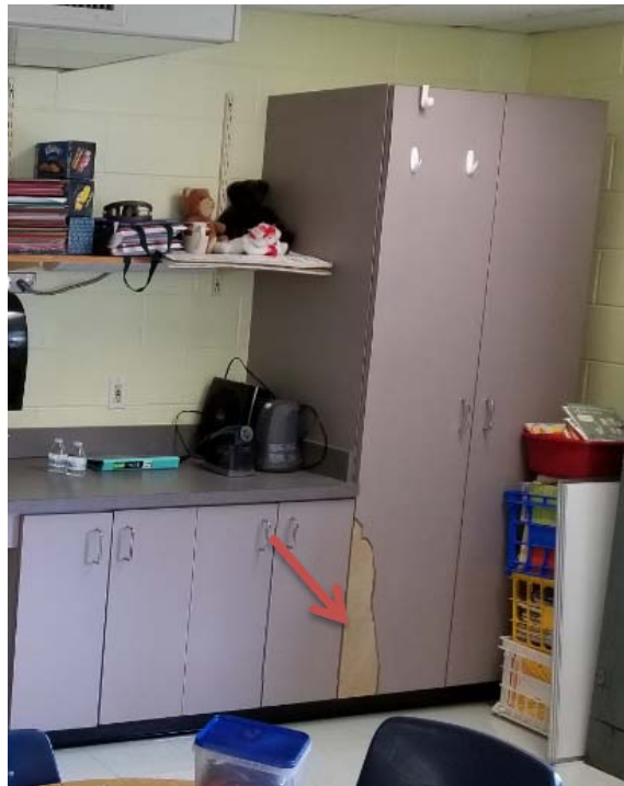
Plastic laminate delamination
