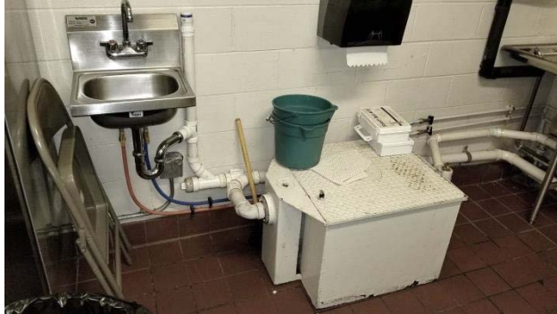
Hand Sink and Grease Interceptor in Kitchen
