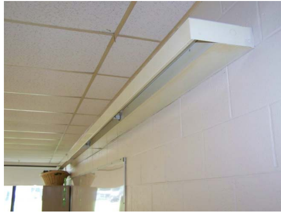
wall mounted classroom lighting fixture with lamps removed
