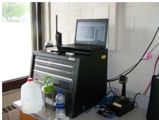
public address system head end equipment
