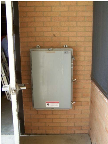
generator connection box
