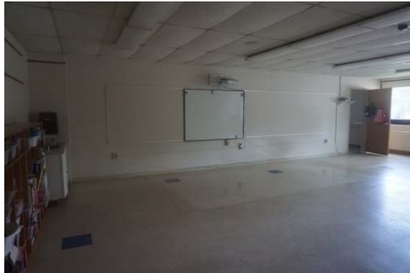
surface mounted raceway in typical classroom
