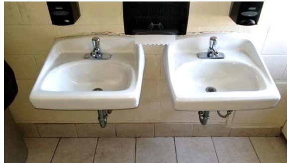
Typical Lavatories with Metering Faucets
