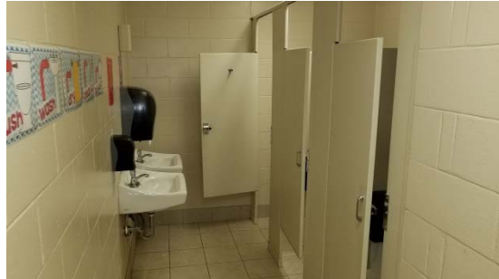
Girls 205 – width from toilet stalls to lavatory wall non-compliant. Similar condition in Girls 108 and Boys 115 and 213.
