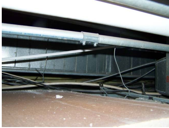
above ceiling first floor, shows wire in conduit, non-metallic sheathed and MC cable
