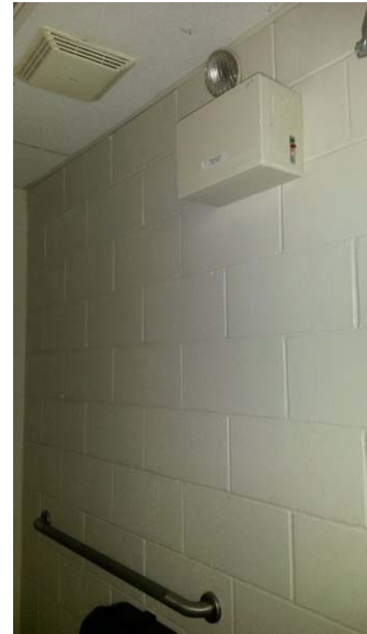
typical emergency egress / life-safety battery unit, this unit has a single head attached
