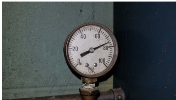
Building Water Pressure Gauge
