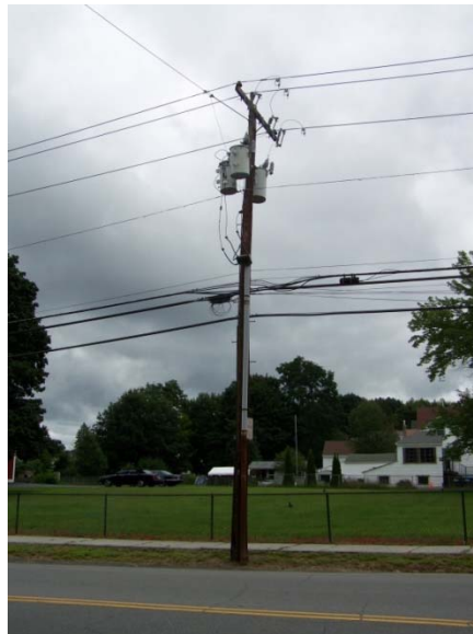
pole mounted transformers serving building
