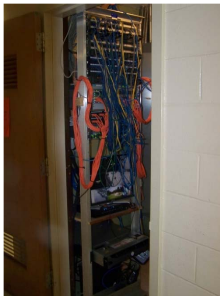
1 st floor, main electrical room, looking left
