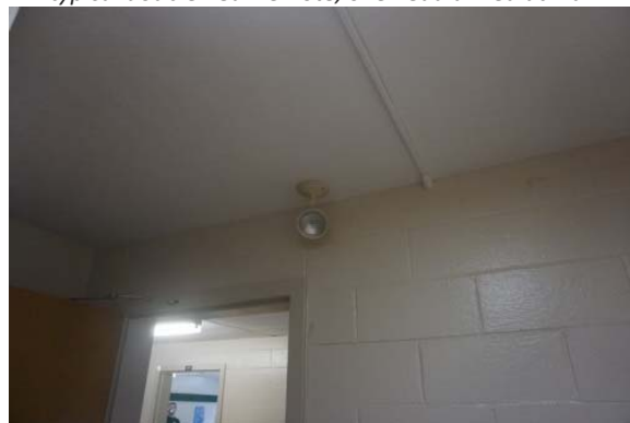
typical single head remote, does not meet NFPA 101 in most cases
