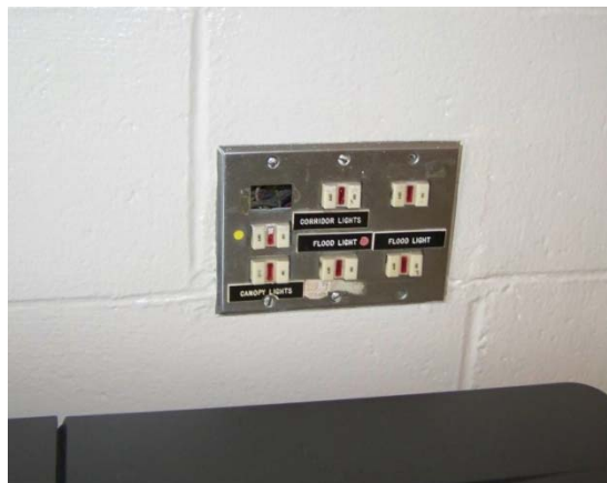
corridor and exterior lighting control station at main office
