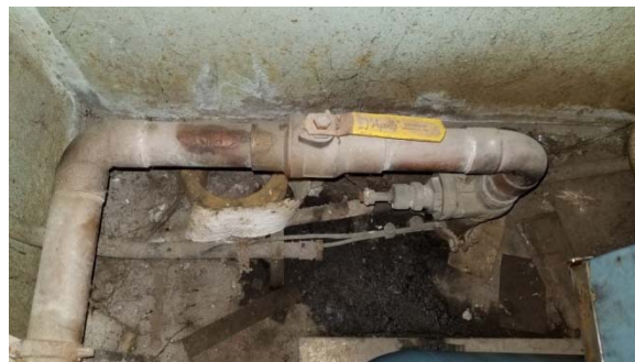
Existing 2" Water Entrance Valves
