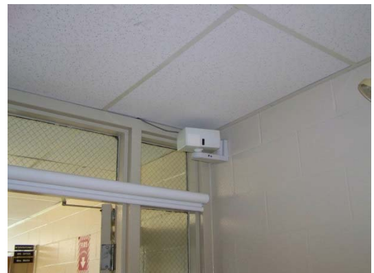
intrusion detection system motion sensor with cabling hanging in space
