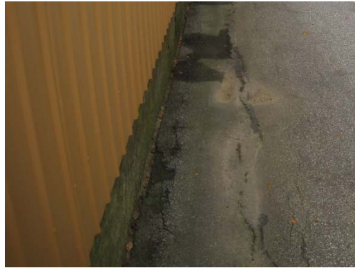
Cracking and differential settlement at north building edge
