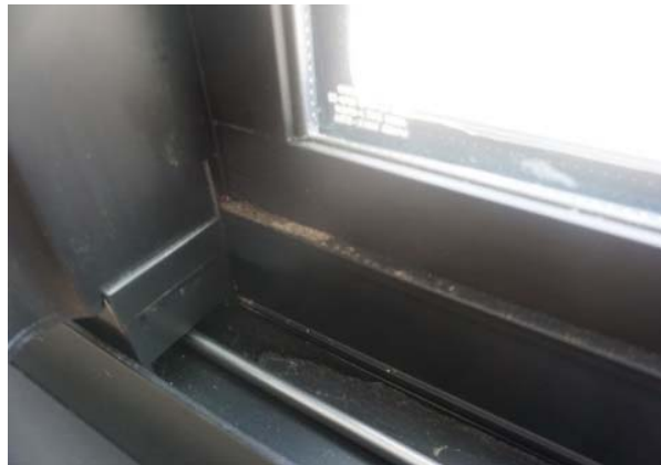
Worn out track
