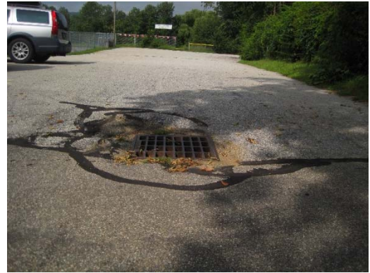
Settlement/sediments surrounding existing catch basin
