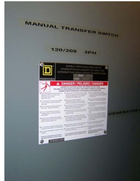
manual transfer switch, close view
