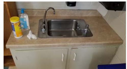
Door replaced with plywood
