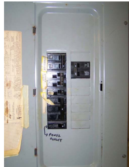
kitchen panelboard #2, surface, space remaining for additional circuit breakers
