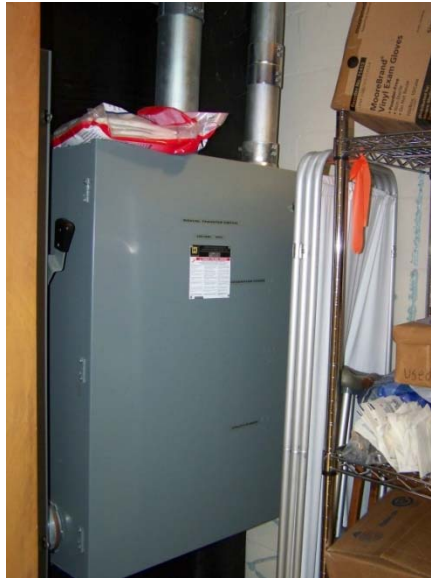
manual transfer switch
