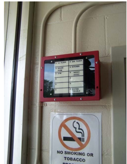
fire alarm system remote annunciator
