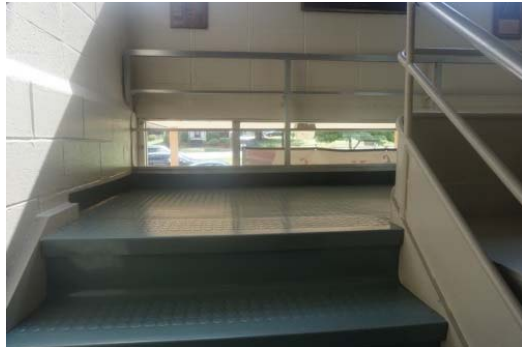
Stair A – guardrail with balusters at landing along open stair does not meet code.
