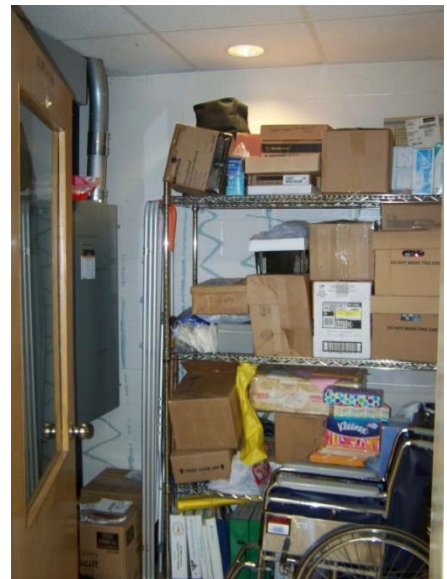
manual transfer switch left side, stored items impede working clearance
