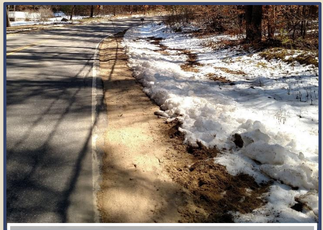
2020 Mar - Roadway Washout, Deerfield Rd
