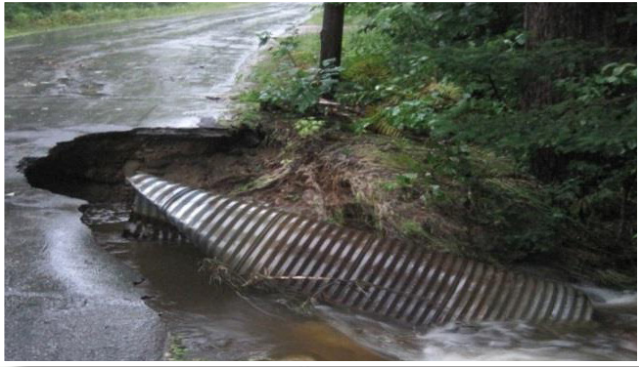
Road washout in Jackson, NH
