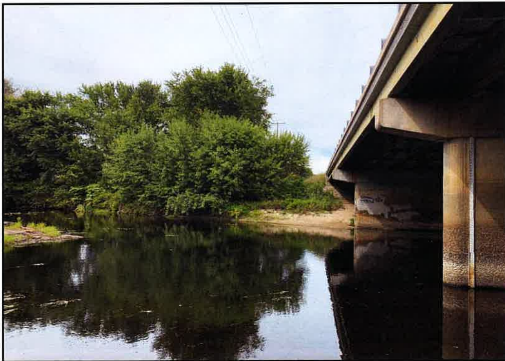
Photo 4: View of northern bank of Suncook River downstream of existing bridge crossing. 9/6/2019.
