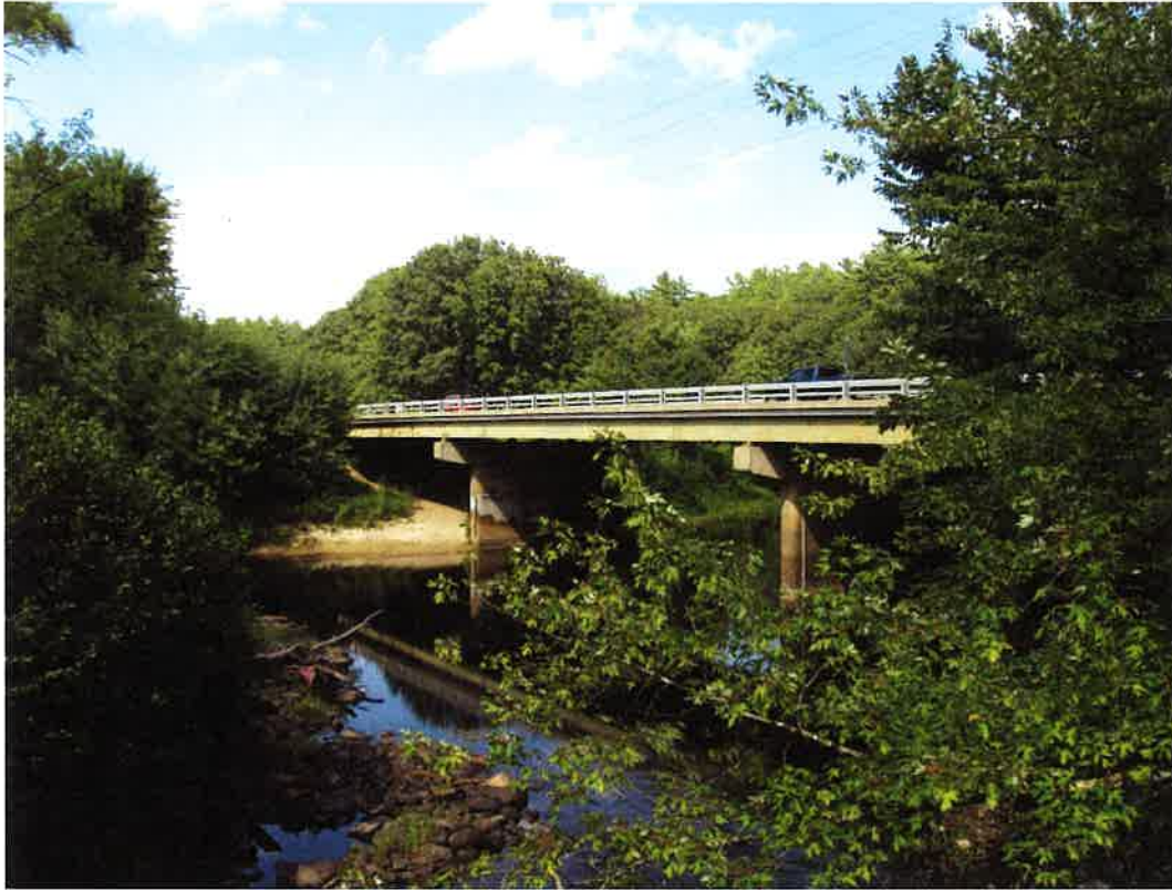
5. View of Allenstown Bridge No. 107/098 profile from the snowmobile bridge, facing northeast. 08/15/2019.
