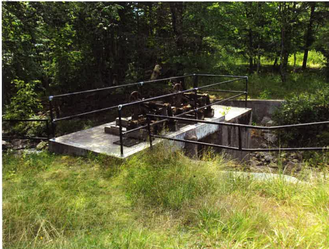
6. View of the former dam penstock controls located south of the current snowmobile trail bridge, facing west. 08/15/2019.
