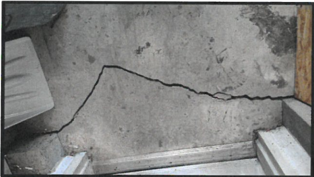
Figure 6 - Exterior Entry Crack
