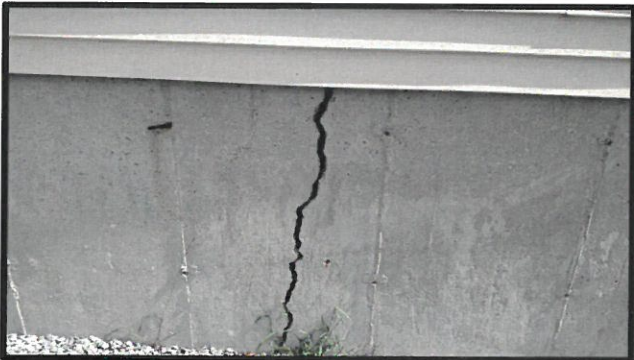
Figure 7 - Structural Crack in Foundation
