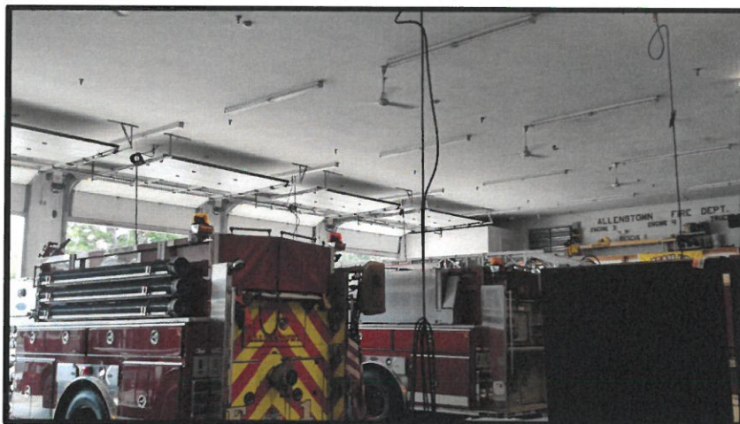
Figure 5 - Apparatus Bays, this picture demonstrates the lack of a diesel extraction system
