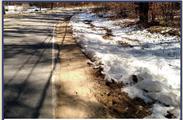
2020 Mar - Roadway Washout, Deerfield Rd Photo courtesy of Paul St. Germaine, Fire Dept
