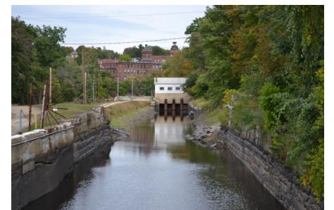
Below: A view of the dam in the China Mill Canal near site location of proposed pedestrian bridge.
