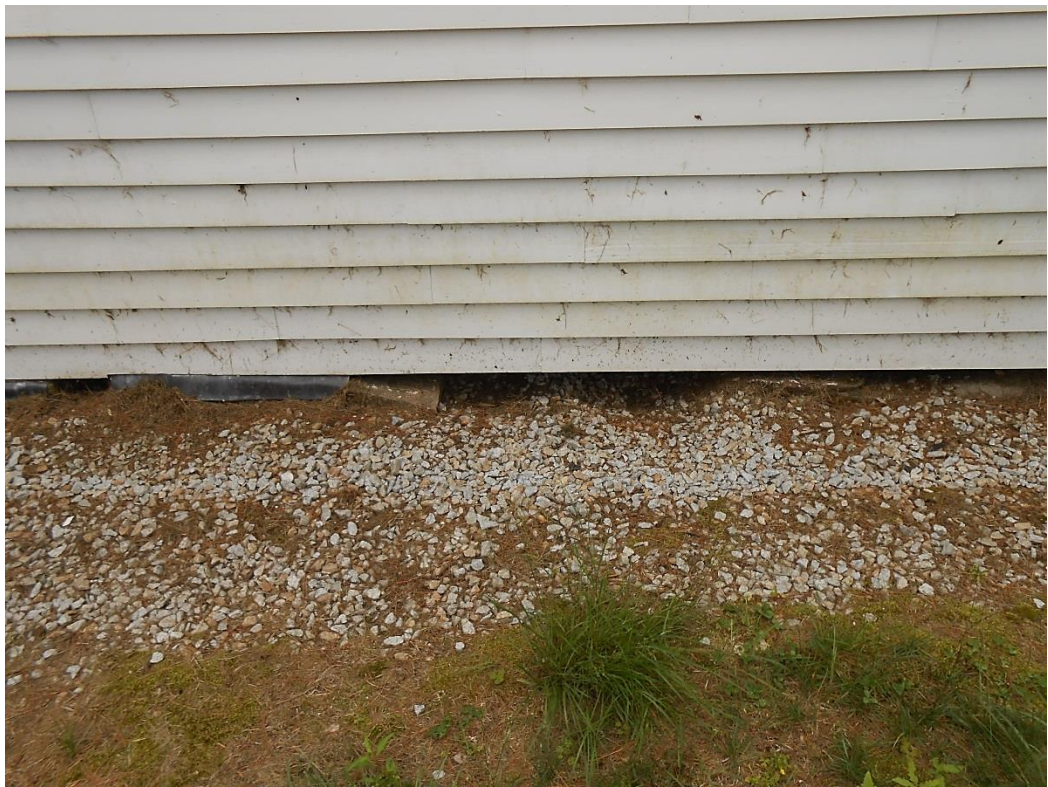
OLD ALLENSTOWN MEETING HOUSE, Rear underpinning, showing access by animals, 8/11/14
